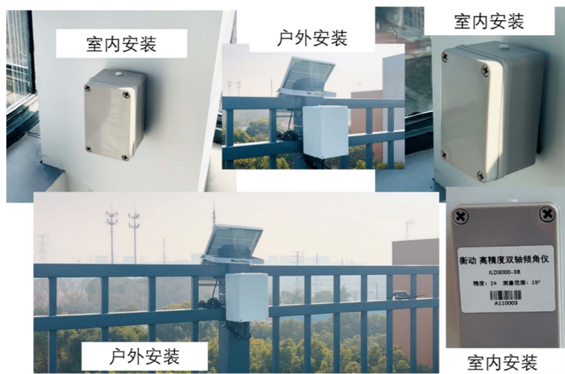
Figure 11. Installation diagram of Low-Power 4G and Wi-Fi stability testing product 图 11. 低功耗 4G 和 Wi-Fi 稳固测试产品安装图片
